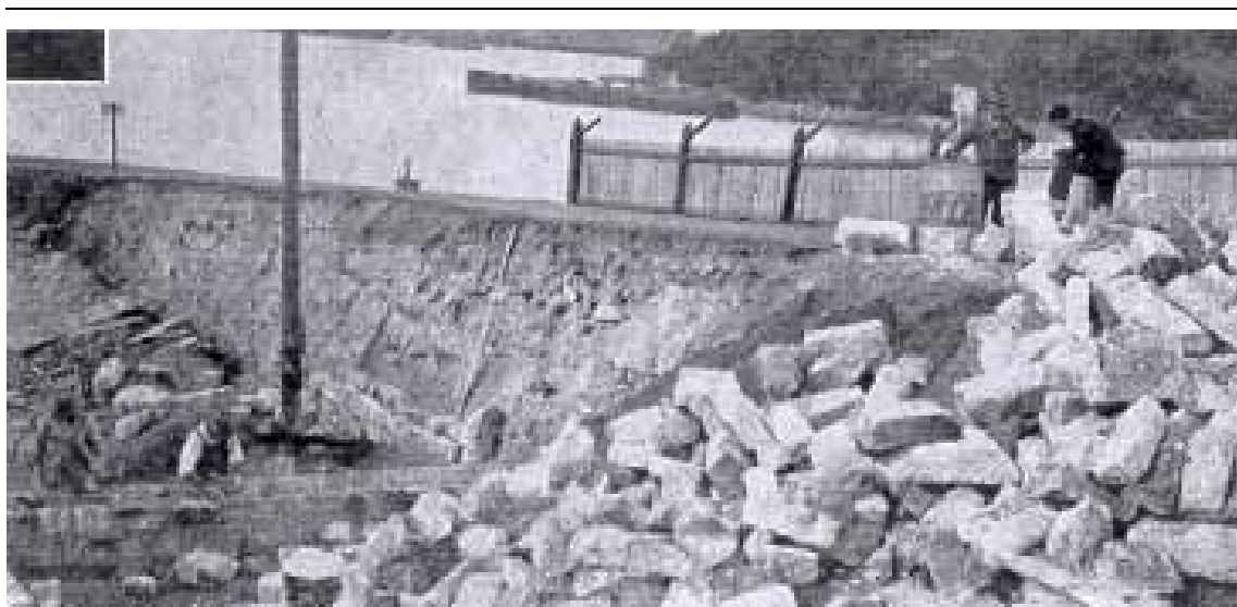
Figure 5.8 The stone store after its demolition in June 1933. The store was demolished to make way for a new storage tank. The stones were reused on site in the construction of a bund wall ('The Accelerator', 1 July, 1936).
