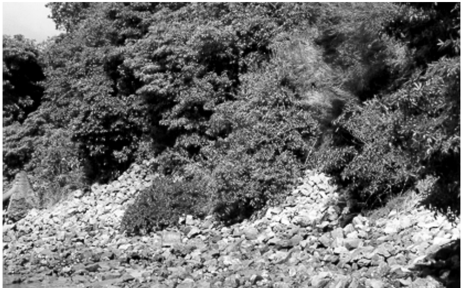
Figure 4.6 The BP site foreshore is substantially modified by land reclamation and stabilisation works.
