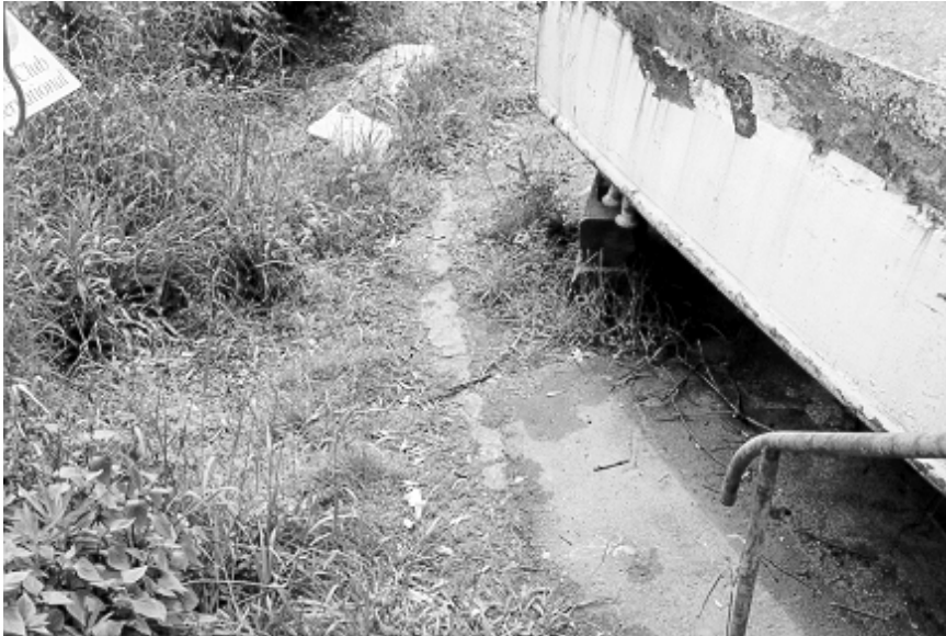
Figure 6.13 Outline of a circular fuel tank, evident at the edge of the bitumen.
