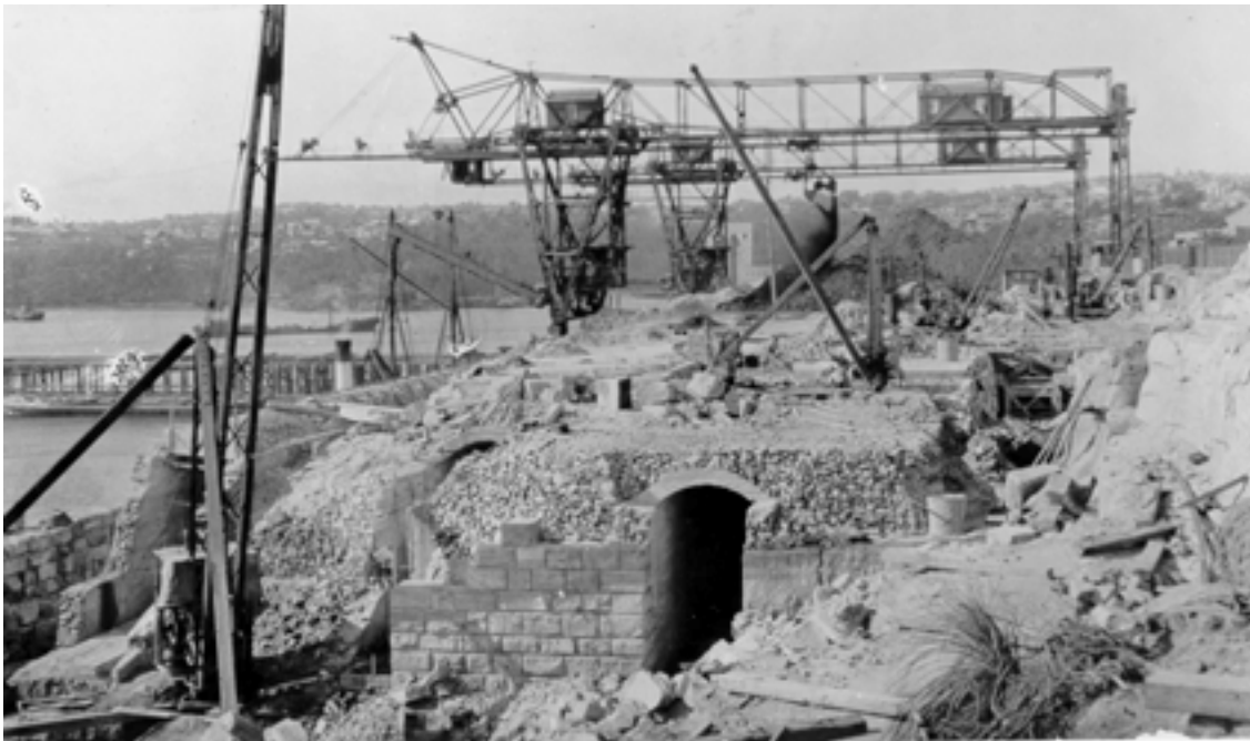
Figure 5.13 Construction of the coal storage tunnels at Balls Head Bay (Stanton Library, PF1239/9).
