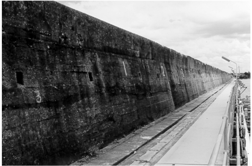
Figure 6.18 Western perimeter wall of Coal Loader platform built from reinforced concrete with Thames River gravel aggregate. Note the base rail for the unloading gantry crane. The numbers correspond to the hoppers in the coal platform floor, and also appear on the eastern wall of the coal platform as well as on the bin gates on the reclaim tunnels. The square holes are air vents into the cellular compartments, between the sea wall and reclaim tunnel No. 1.
