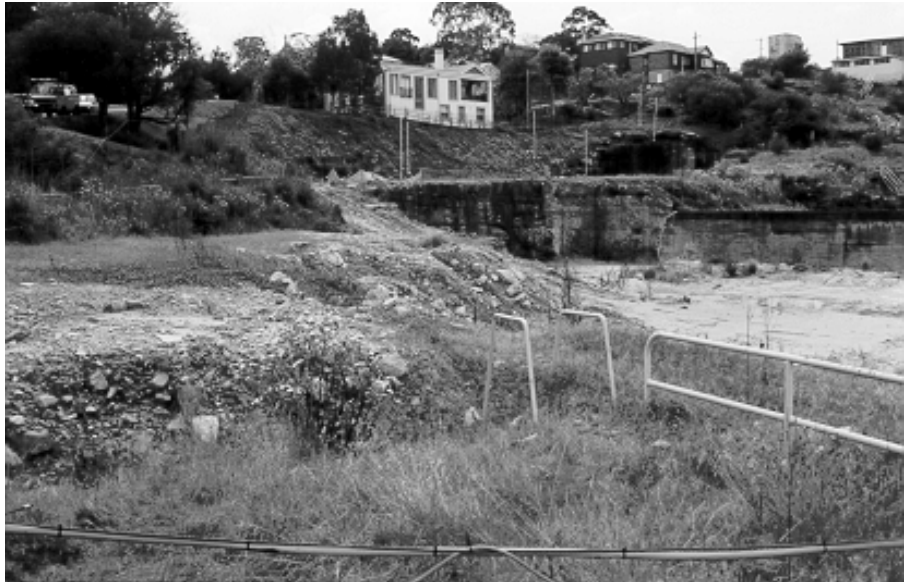
Figure 4.1 The BP site, southwest corner, showing the extent of cut and fill activity.
