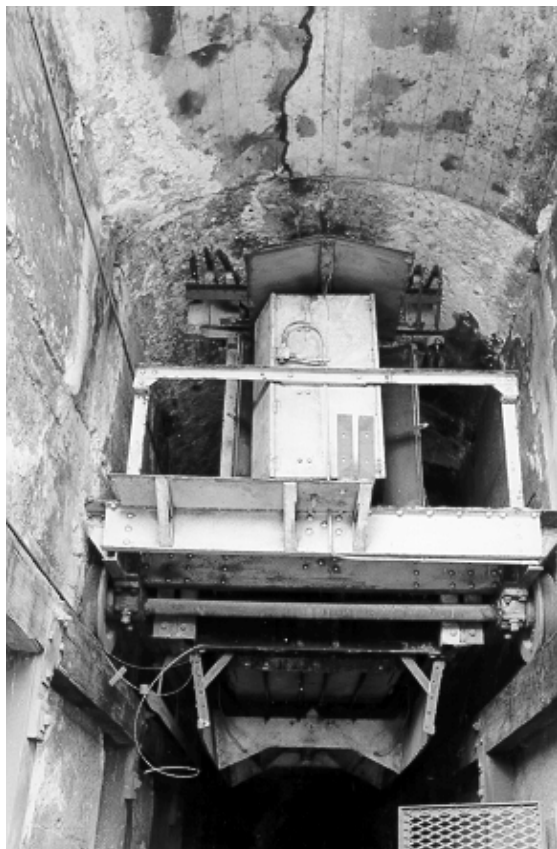
Figure 6.22 Mead Morrison travelling feeder, in situ in tunnel No. 1. The Mead Morrison equipment was purchased second-hand, installed c1921, and operated until 1976.
