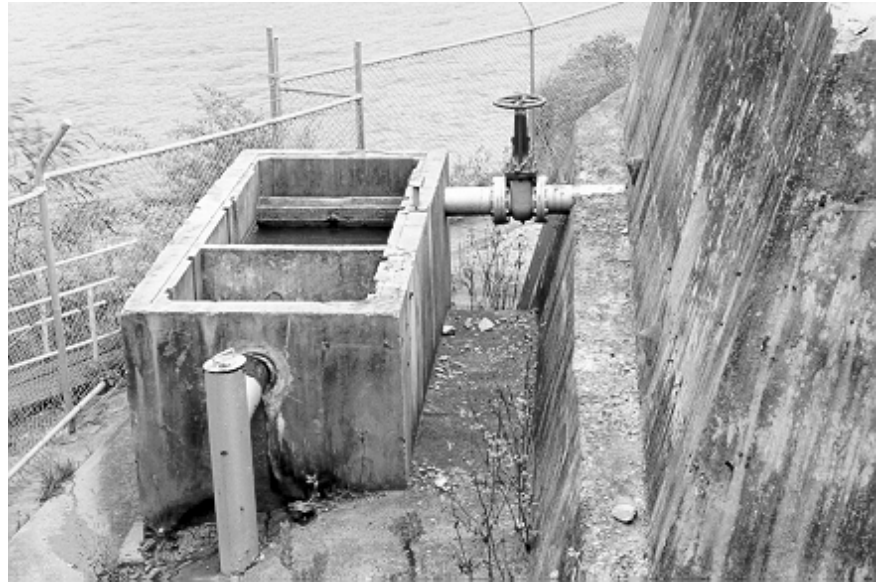
Figure 6.10 Concrete tanks with weirs, baffles and valves provide evidence of the methods used in the transfer of fuel and water at the BP depot.
