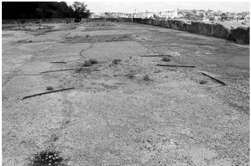
Figure 6.19 Square, backfilled recessed hoppers in Coal Loader platform floor. There are thirty-three hoppers. Note the deteriorated condition of the perimeter wall.
