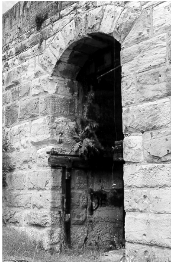
Figure 6.21 Northern entrance to reclaim tunnel No. 1 faced with large sandstone blocks. Note the timber post and beam, to support the steel rail for the Mead Morrison travelling feeder.
