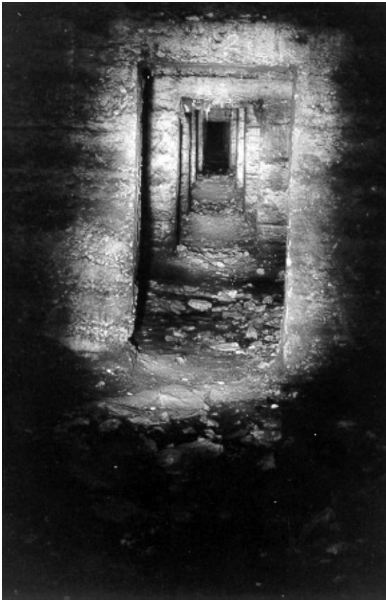
Figure 6.20 Interconnecting doorways between areas in the cellular section, behind the sea wall of the Coal Loader platform. These compartments extend the length of the structure, and are mainly built from formed concrete and aggregate.
